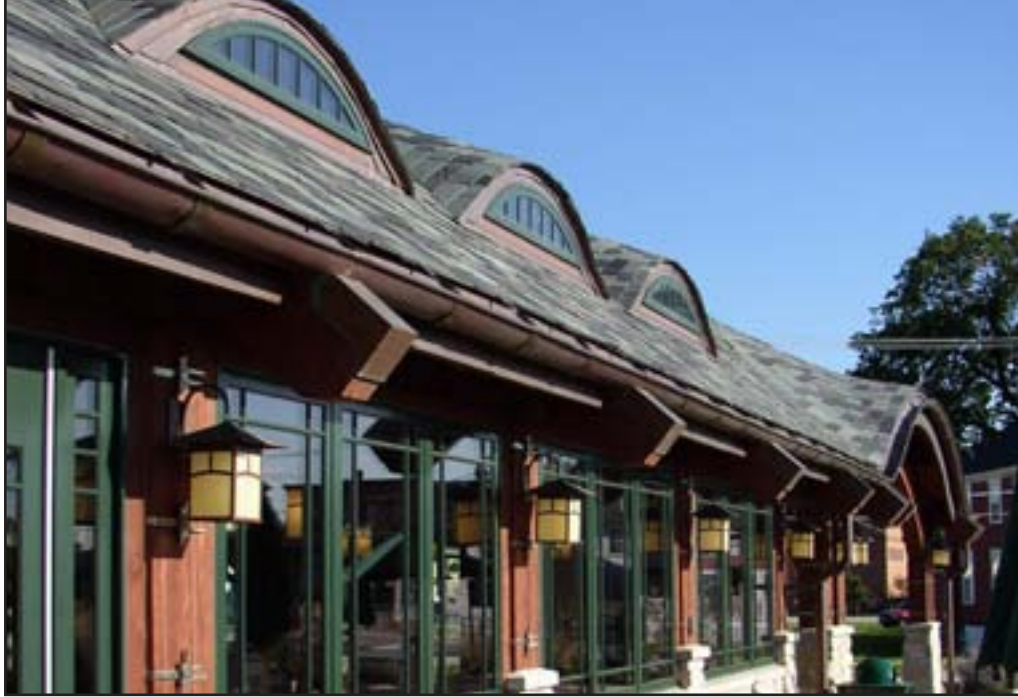
LEFT AND BELOW: Although the eyebrow dormers and arches provided a challenge for the slate roofers, the Tinley Park station project went off without a hitch.
